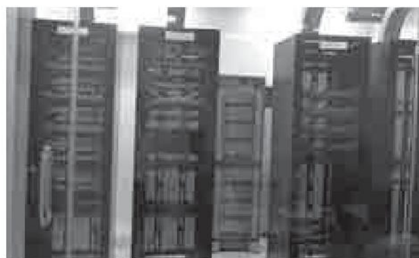
The Data Center of MIS
